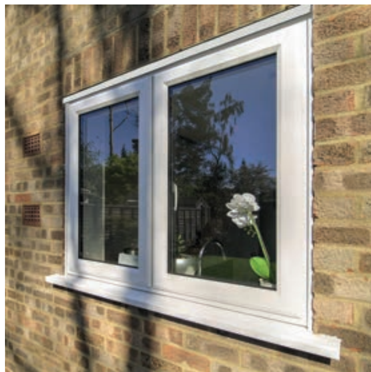
Concealed Ventilation installed through the outer frame
